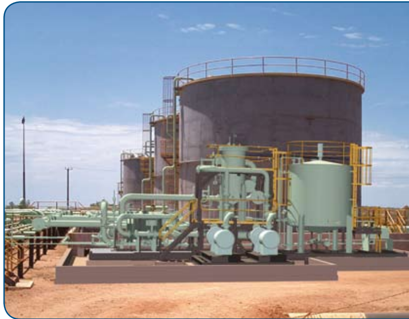
The PWFS fabricated for Chevron's Barrow Island's central processing facility.
