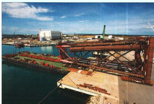
SIGNIFICANT STRUCTURE: The multi-million dollar Blacktip wellhead platform at the Australian Marine Complex in Henderson.
